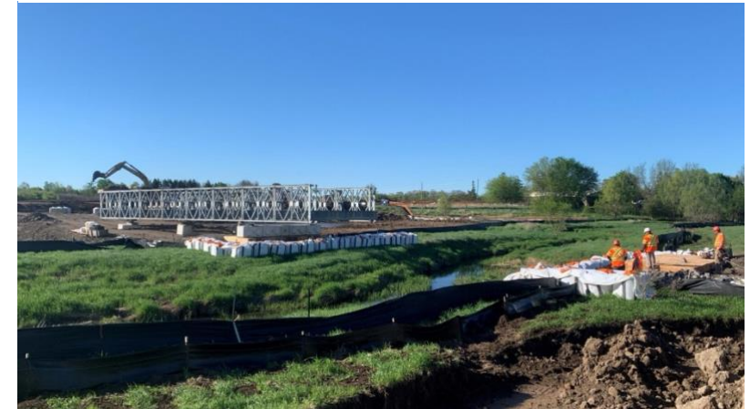
Temporary bridge installation with erosion control and wildlife fencing in place. May 17, 2022
