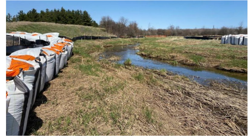
Temporary Indian Creek crossing with pea gravel bags and abutment foundations. April 28, 2022
